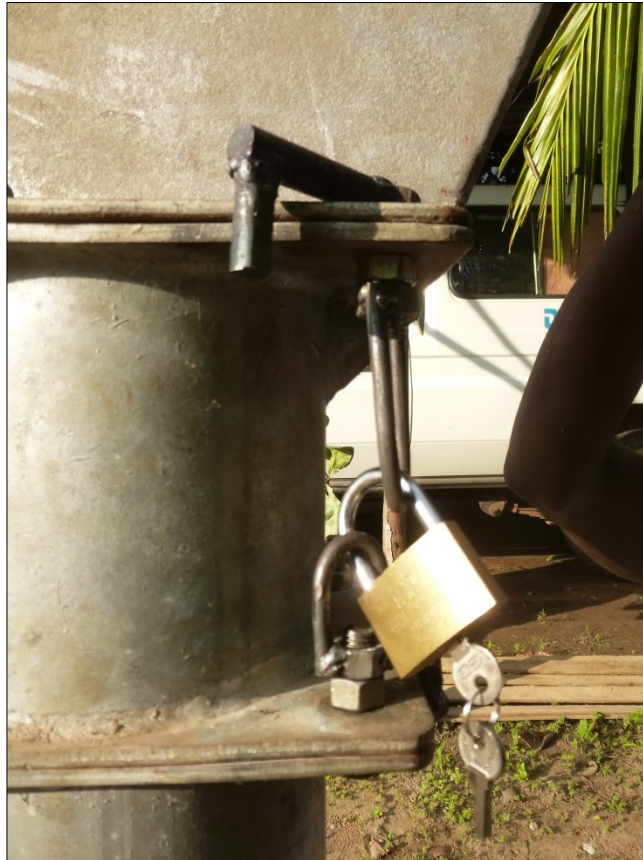
A 90° leg has been welded to the original bolt (Top). It is therefore not possible to rotate the bolt and unscrew the nut beneath. (the lower bolt has also been modified but it is not visible on the photo. It is identical to the top bolt.) The top and lower nuts have been modified with a U flange being welded on each of them. They can therefore be linked together with a padlock.
